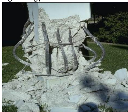
Figure 1: Failure at Construction Joint
